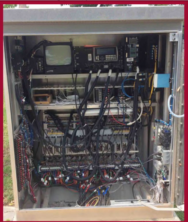
Coordinated Traffic Signal System
